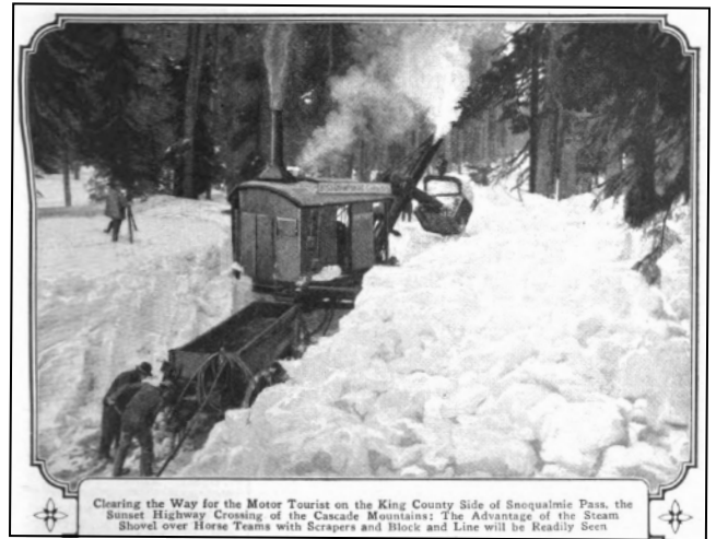
Clearing the Way for the Motor Tourist on the King County Side of Snoqualmie Pass, the Sunset Highway Crossing of the Cascade Mountains: The Advantage of the Steam Shovel over Horse Teams with Scrapers and Block and Line will be Readily Seen
