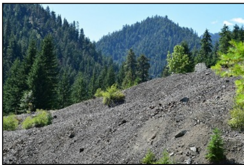
Landslide on old Ingall's Creek Roadbed - YT Route
