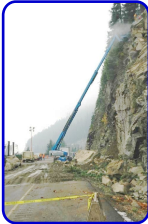
Work just started to bring down loose rock and "bolt" the rest in place.
